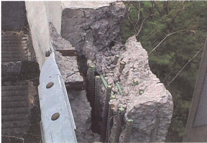
COLLISION DAMAGE APPROACH #2 LEFT SIDE WITH EXPOSED REBAR
